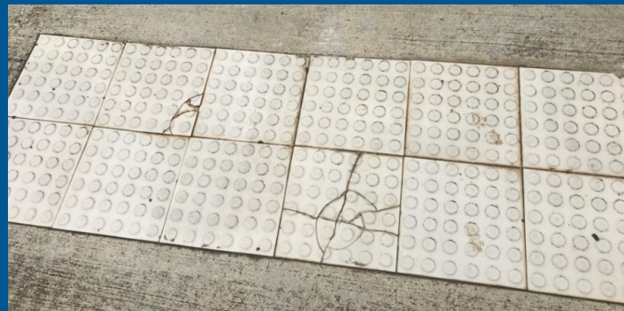
Damaged Existing Ceramic TGSI
