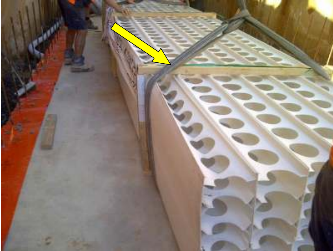
Photo No: 3 – Choked Crane Sling Damaging Webs
